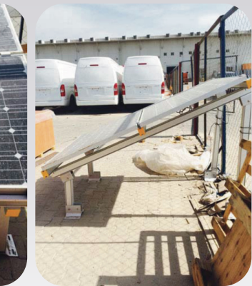
End user: Dubai Municipality Location: Dubai 5kwpc, Solar off - grid system
