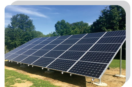
GROUND MOUNTED SYSTEM
