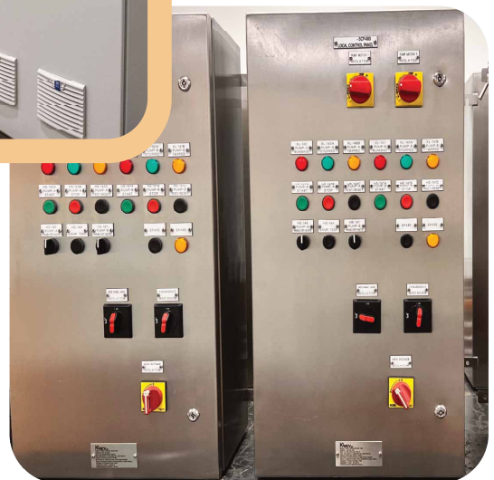
Local Control Panel
